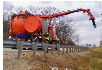
MCDOT vacuum truck
