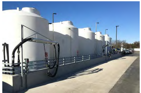
View of MDCOT liquid brine tank farm with secondary containment
