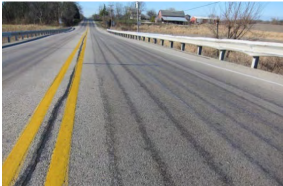
Striping on road from liquid “anti-icing” application
