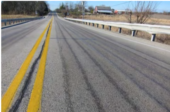
Striping on road from liquid “anti-icing” application
